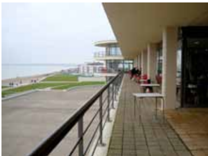
Above: DLWP balcony and Solarium area on the First Floor Level. These areas are fully exposed to the impacts of the marine environment.
